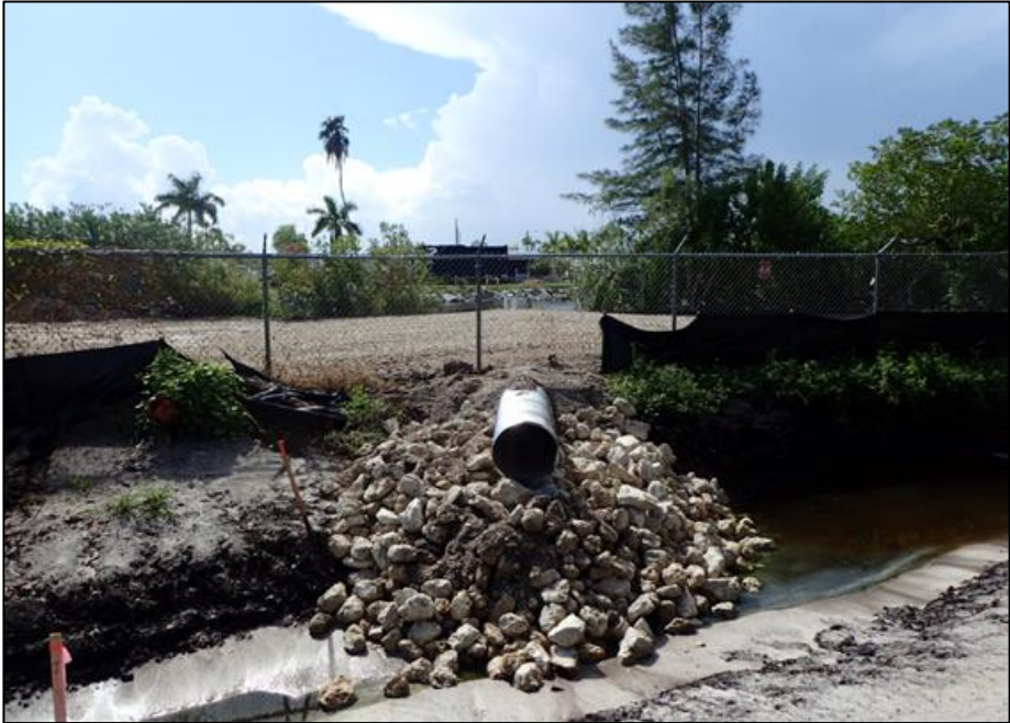
Figure 16 – Installation of pipe connecting off-stie borrow pit to created wetland at FISH Preserve Phase IV restoration project
