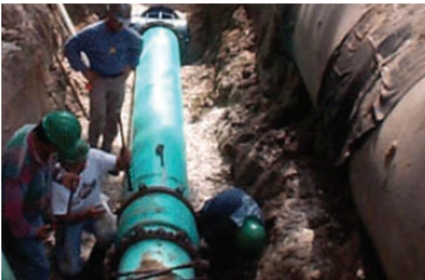
Installation of sewer main, Lockwood Ridge Road, Sarasota County. (Hazen & Sawyer Environmental Engineers)
